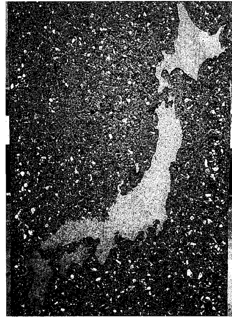
Photo 6 骨材あらわし仕上げの事例 Concrete Surface of Exposed Aggregate Finishing
