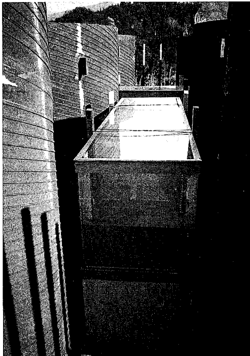
Photo 1 橋脚頂部に設置した重泥水TLD Heavy Mud TLD Installed on Top of Pier
