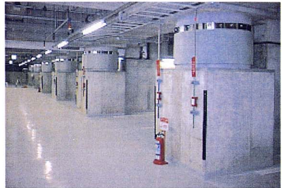
Photo 5 耐火被覆取り付け事例 Schematic of Installed Fire Protection System
