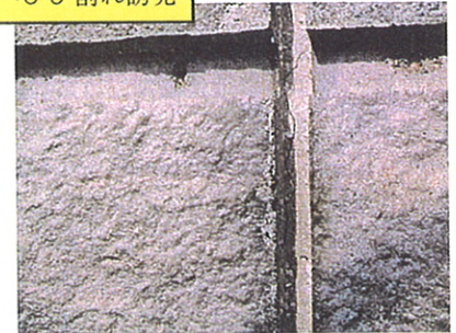
Photo 4 目地へのひび割れ誘発 Induced Cracks along Joiners
