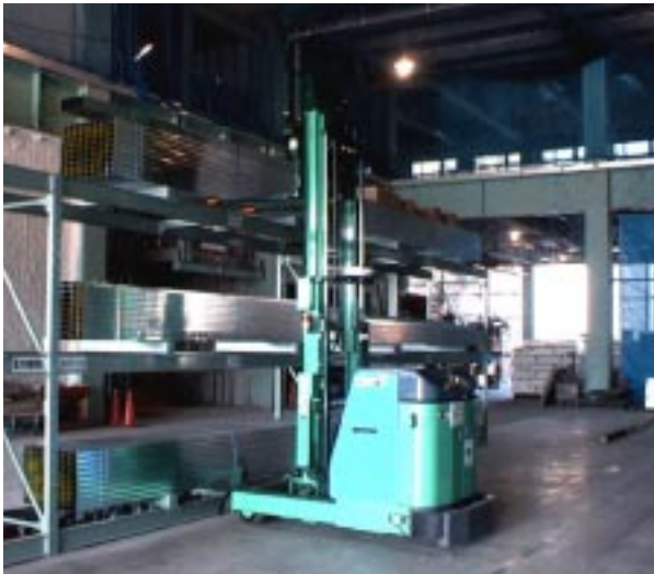
Photo 1 A G F と立体ラック棚 Automatic Guided Fork-lift and Solid Rack
