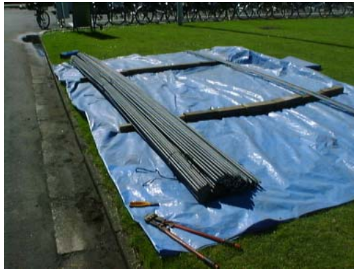
Photo 8 搬入時の未加工鉄筋束 A Bunch of No Processing Reinforcing Rods
