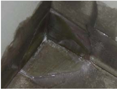
Photo 2 FRP成形役物の張付け Waterproofing with a Preformed accessory made from FRP
