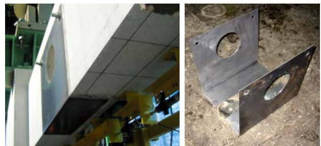
Photo 1 補強状況 View of Strengthening Portion Photo 2 折り曲げ鋼板 Bending Steel Plate
