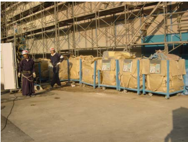
Photo 1 廃棄物置き場の状況 (中小規模現場) Construction Waste Yard (Small Construction Site)
