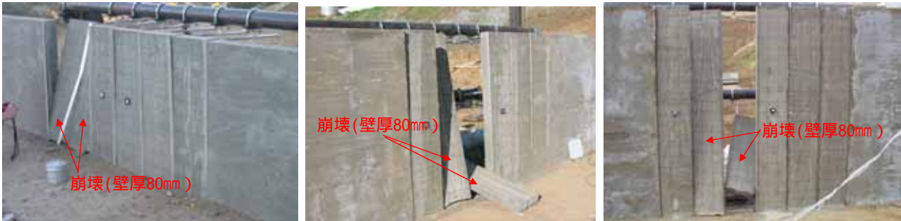
Photo 4 損傷状況(壁高さ1m) Damage of 1m-Height Walls
