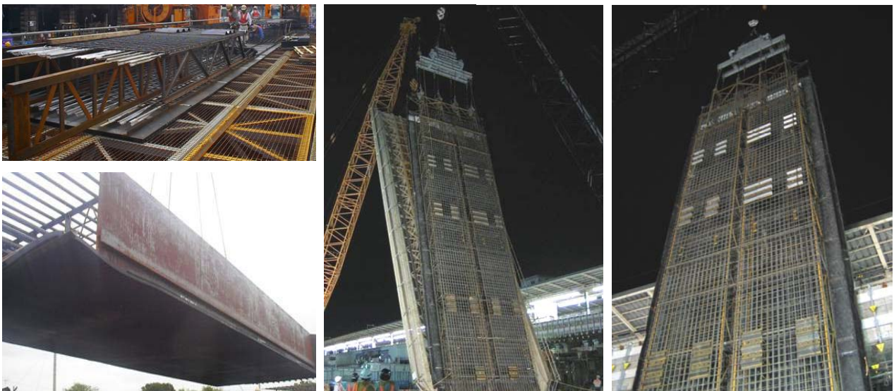
Photo 2 防振ゴムパッド付き鉄筋かごの組立・建込み状況 Setting of Isolated Underground Wall
