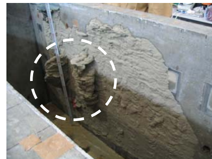
Photo 7 土水圧を考慮した注入試験(ケース3) Situation of Injection Test Used Medium Soil Tank Considered Soil and Water Load (Case3)
