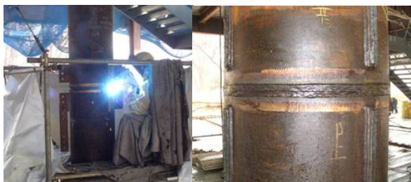
Photo 5 鋼管柱継手の現場溶接状況 Onsite Welding of Joint of Steel Pipe Column
