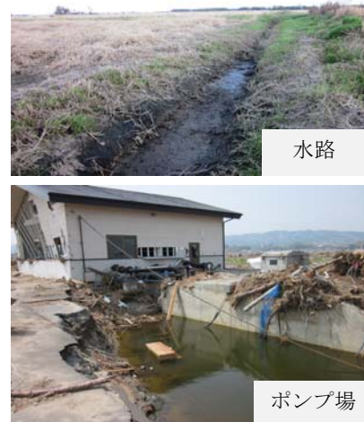
Photo 3 被害を受けた水路・施設 Tsunami-affected a waterway, drainage pump station
