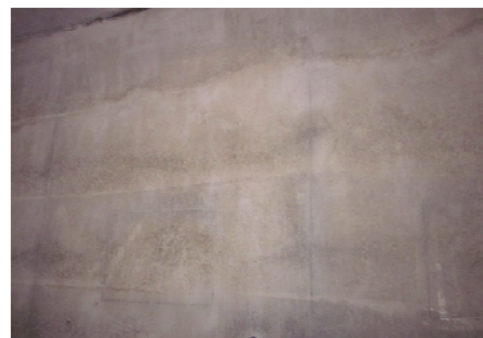
Photo 9 側壁部に生じた打重ね線の例 Example of Layer Streaking Occurred at Sidewall
