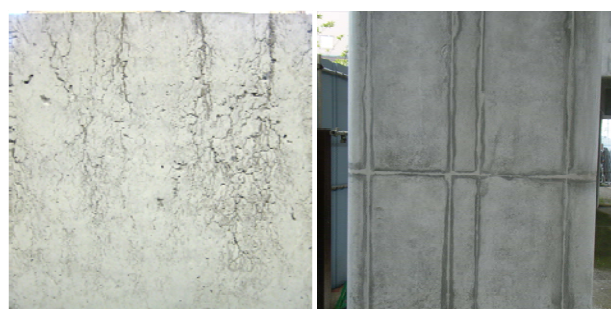
(a) 鉛直面に生じた砂すじ (b) 型枠の継目に生じた砂すじ At Vertical Plane At Joints of Forms
