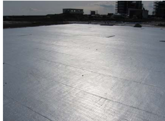
Photo 3 床スラブへの養生シートの敷設状況 Situation of Covering of Cure Sheet to Floor Slab
