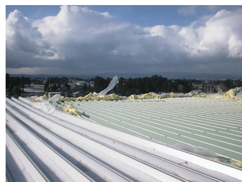
Photo 18 二重折板屋根の飛散事例 Scattering of Double Folded-Plate Roof
