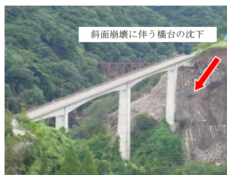
Photo 1 阿蘇長陽大橋の被害 Damage of Aso-Choyo Great Bridge
