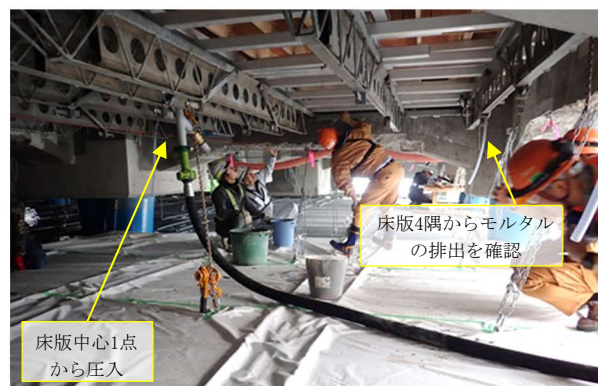
Photo 8 栈橋床版下面への圧入状況 Situation of Press-fitting Underside of Pier
