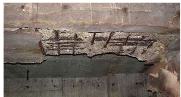
Photo 1 栈橋下面の塩害による劣化の例 Example of Salt Damage on the Underside of the Pier
