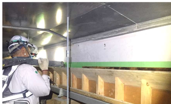
Photo 9 栈橋梁部下面の打込み状況 Placement Status of the Beam Part
