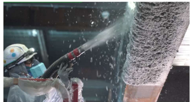
Photo 1 技能工による吹付け状況 Spraying Situation by Worker of Fireproof Coating
