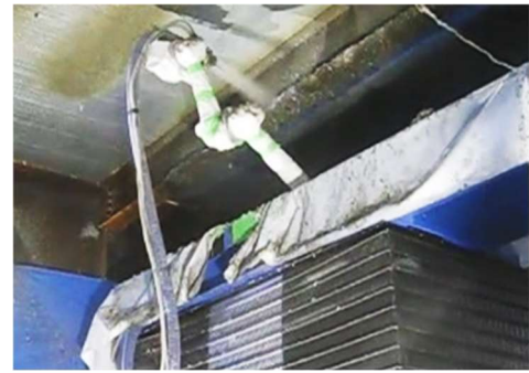
Photo 7 耐火被覆の吹付け状況(下フランジ) Fireproof Coating Spraying by Robot (Lower Flange)
