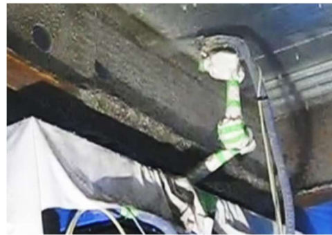
Photo 8 耐火被覆の吹付け状況(ウェブ) Fireproof Coating Spraying by Robot (Web)
