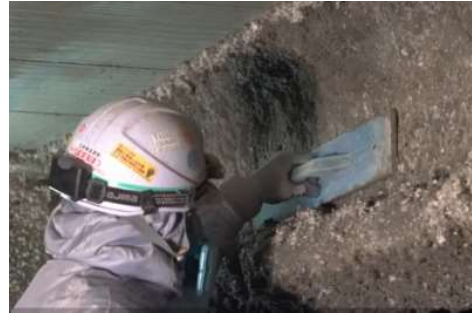
Photo 4 技能工によるコテ押さえ状況 Pressing Situation by Worker of Fireproof Coating
