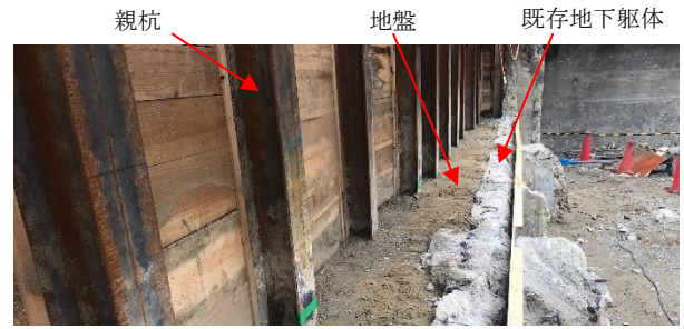
Photo 2 親杭・既存地下外壁間の地盤 The Soil between Soldier Beams and Existing Underground Exterior Walls
