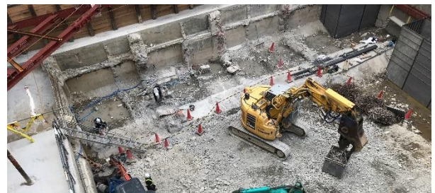
Photo 3 既存地下躯体の最終解体状況 Final Demolition of Existing Underground Structures
