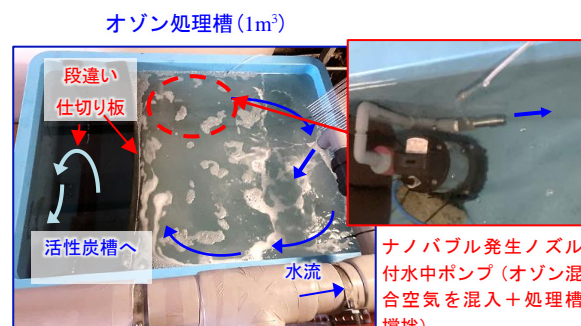
Photo 3 実証施設のオゾン処理槽 Ozone Treatment Tank at the Demonstration Facility
