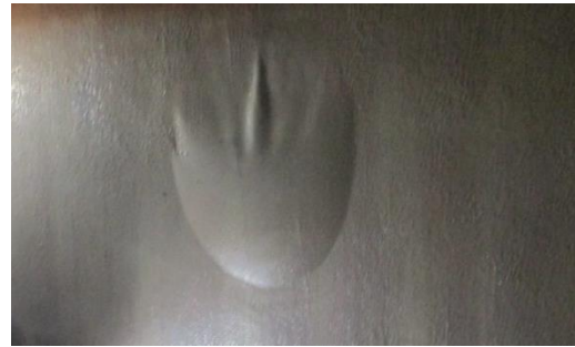
Photo 1 背面水圧による防水層の膨れ Blistering of the Waterproof Layer due to Backwater Pressure
