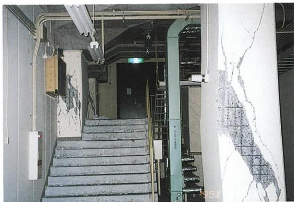
Photo 1 上沢駅C断面の被害状況 Damage of C-cross Section at the Kamisawa Station
