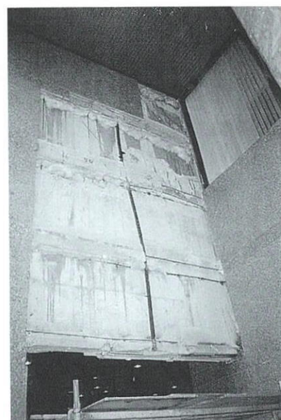
Photo 9 湿式石張りの被害 Damaged Stone Finish
