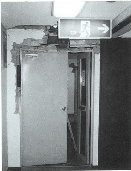
Photo 13 鋼製避難扉被害例 Damaged Steel Door for Fire Escape
