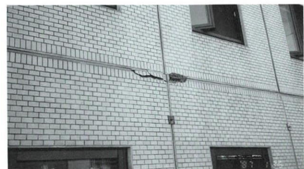
Photo 3 目地周辺の版の損傷 Damaged Panel Around Joint
