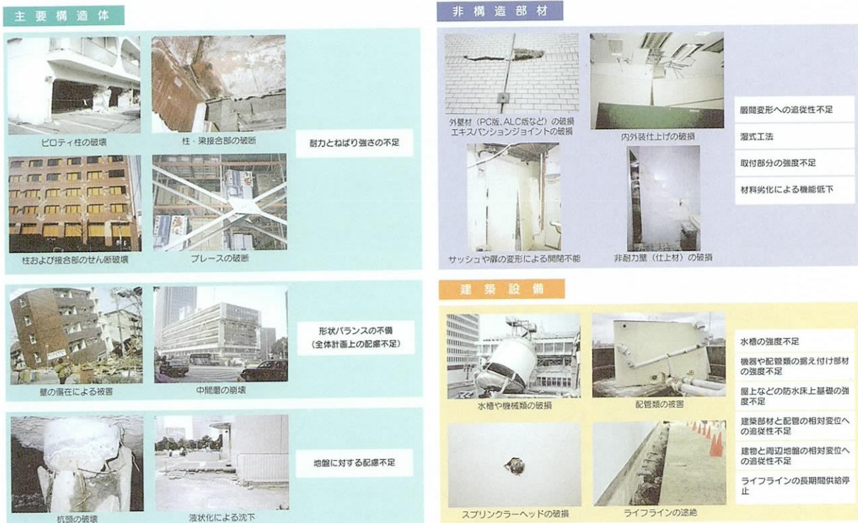
Fig.1 阪神・淡路大震災の被害と原因 Earthquake Damages and Causes
