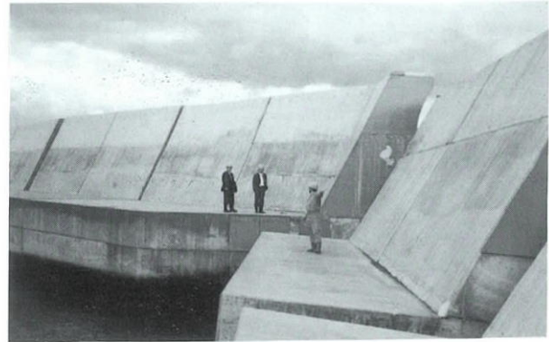
Photo 1 被災状況 (P.I. II 西・南護岸) Damage to Revetment (No. 1)
