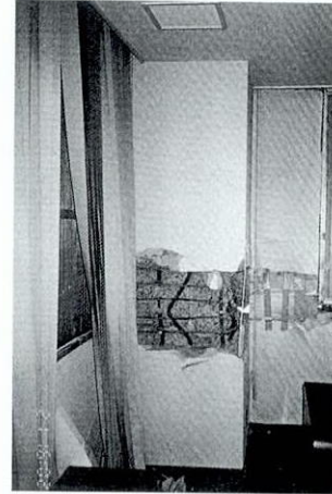
Photo 7-1 柱の損傷 Damage of RC Column
