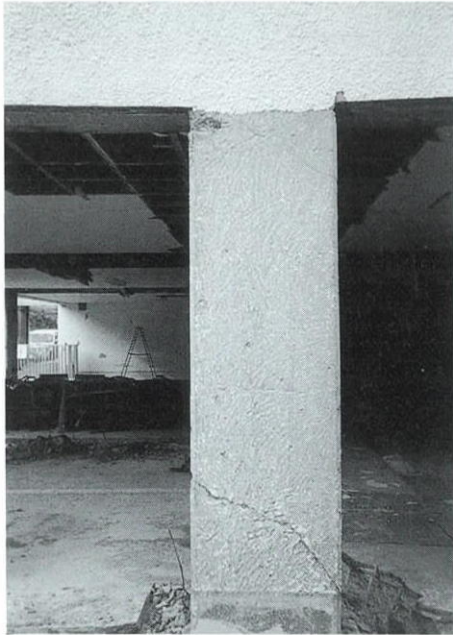
Photo 2 1階①-C柱せん断ひび割れ Shear Crack of ①-C Column
