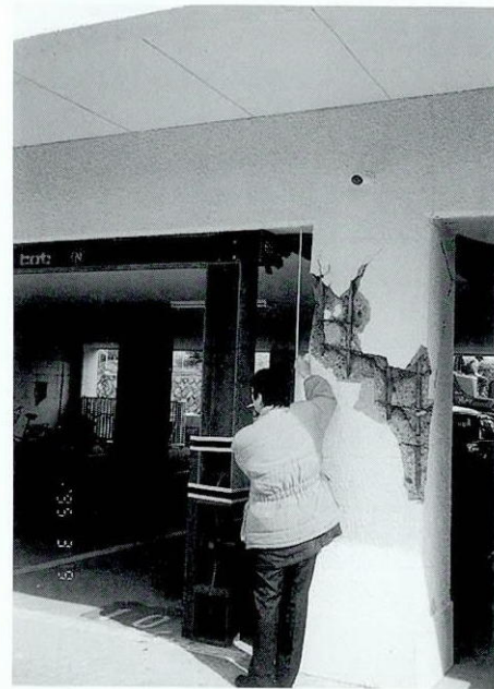
Photo 1 1階③-B柱の破損状況と仮設鉄骨支柱 Damage and Steel Support of ③-B Column on 1F
