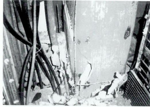
Photo 11 柱部破断 Cracking of Column
