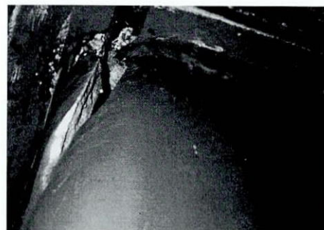
Photo 8 Bビルの仕口内への破断 Cracking into Beam-to-Column Connections
