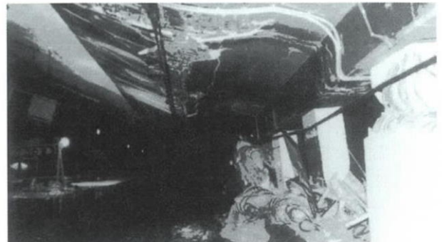
Photo 2 地下鉄駅舎の被害状況 Severe Damaged Underground Subway Station
