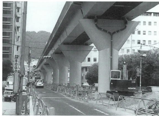
Photo 1 新交通システム復旧状況 General View of Retrofit Work of New Transit Line
